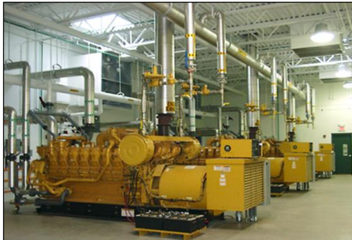
Landfill gas-to-electric engine room (Elk River Municipal Utilities)
