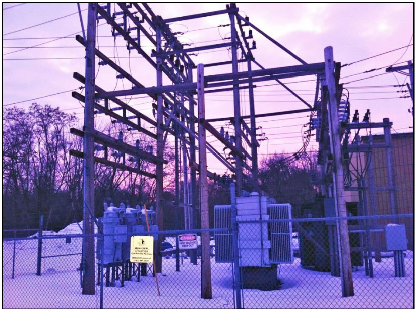
Power Plant Substation (Elk River Municipal Utilities)
