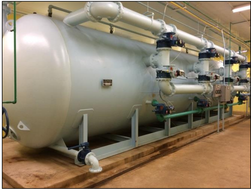
Filter at Well No. 7 Building (Elk River Municipal Utilities)
